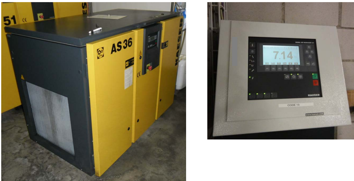
Figure 8 One air compressor (left) and display of new, higher-level control system (right)
